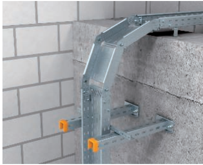
Installation of falling adjustable vertical bend Adjustable vertical bend to bridge height offsets. The adjustable vertical bend is connected with to the cable tray using the adjustable connectors.
